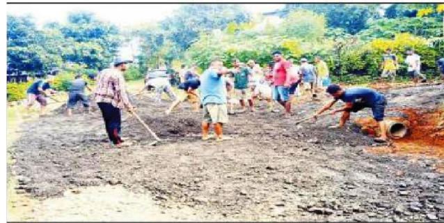
The Keileilwa Colony Ward No 6 social work in progress at Jalukie Town.
